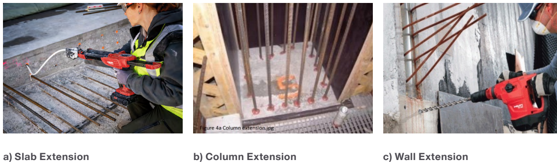
Fig. 2.3: Examples of extension of R.C. elements with lap splices using post-installed rebars
